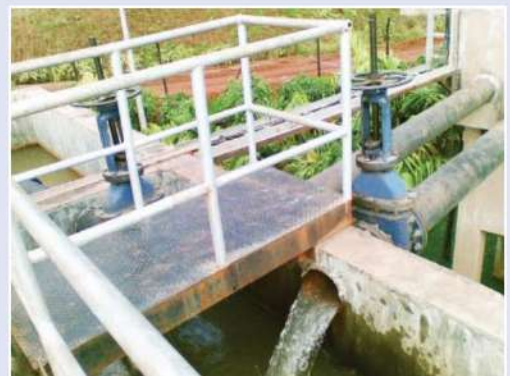
GATE VALVES IN OPERATION AT A WTP
