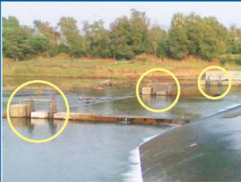
1200 MM SLUICE VALVES AT A BARRAGE
