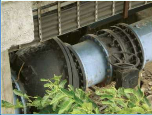
MULTI DOOR NRV & BF VALVE AT RAW WATER PUMP HOUSE
