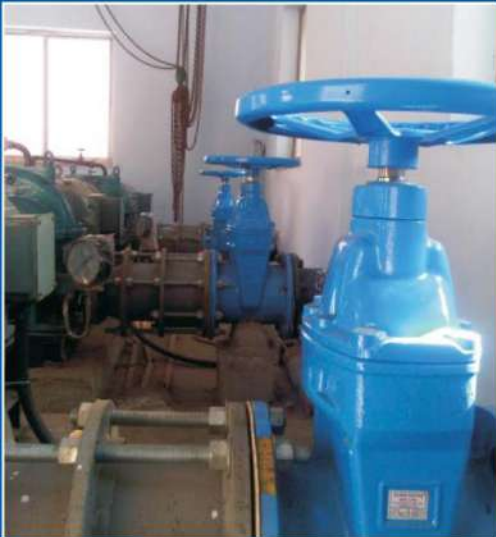
DI RESILIENT SEATED GATE VALVE AT A PUMP HOUSE
