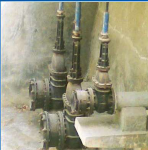
RISING STEM GATE VALVES AT STORM WATER SITE
