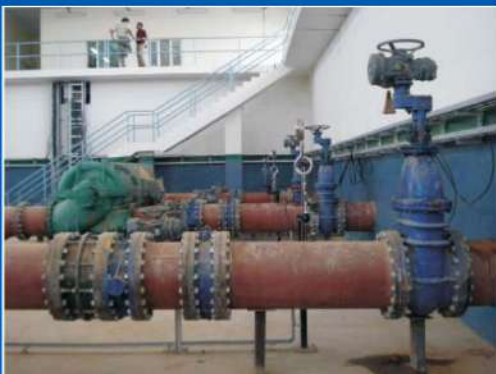
EOP SLUICE VALVE, DUAL PLATE CHECK VALVE AND BF VALVE
